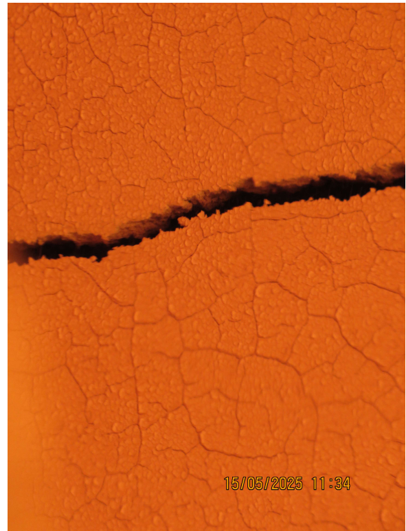
Figure 10: Horizontal crack 34 minutes after the start of the test.
