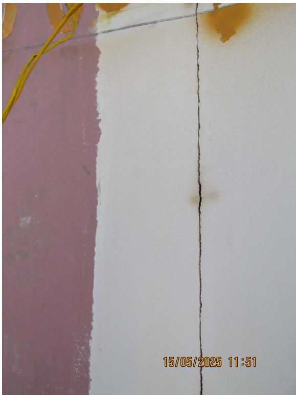
Figure 11: Vertical crack on un-exposed surface 51 minutes after the start of the test.
