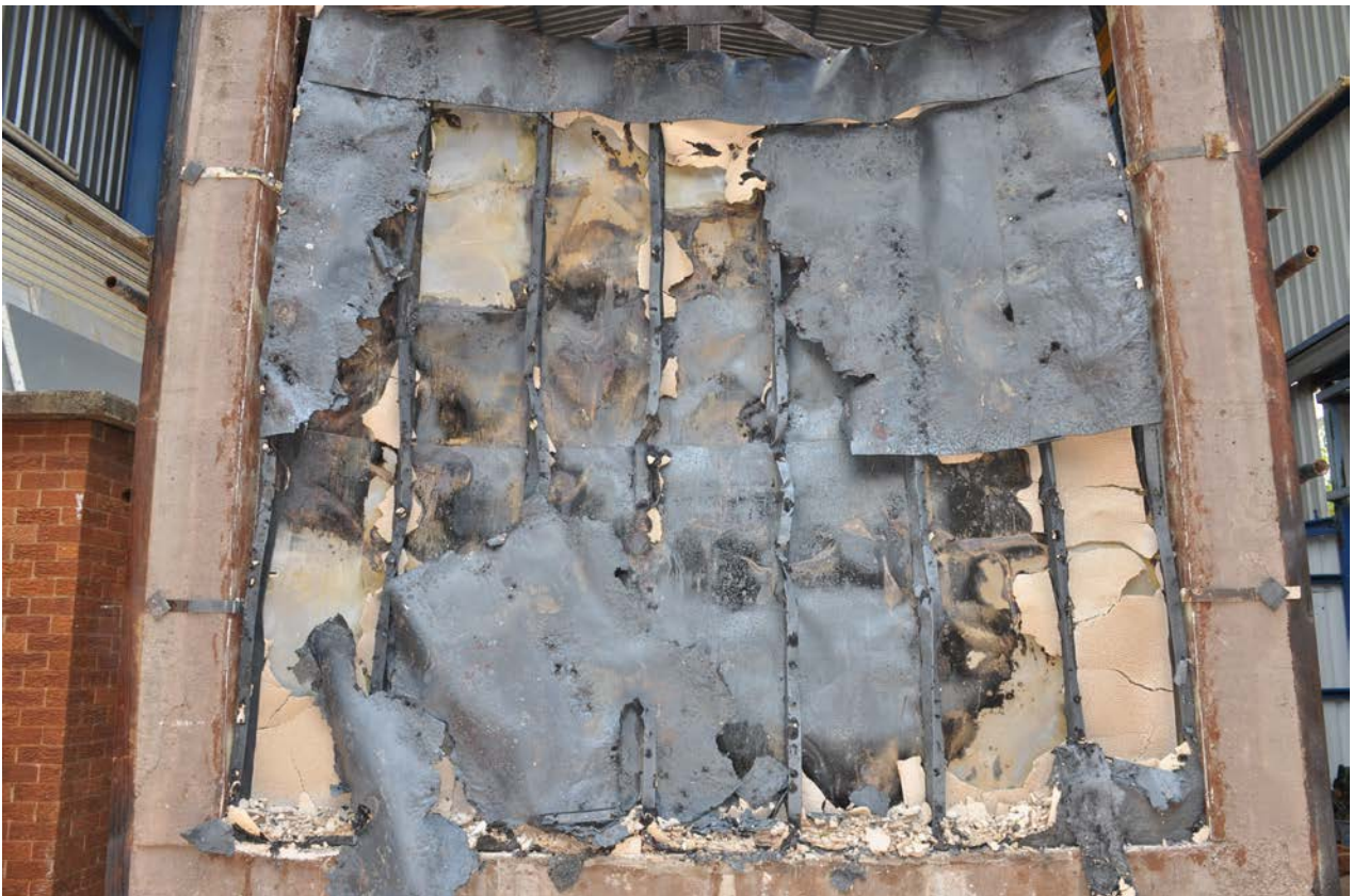
Figure 1.2: The exposed side of the system after the test conclusion
